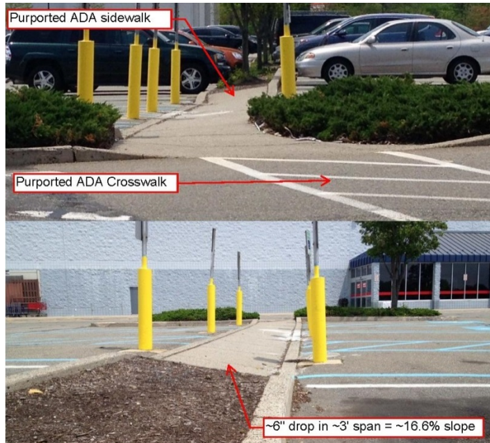
Figure F-11 (Picture of Apparent ADA Non-Compliance in Longitudinal Island Sidewalk)
