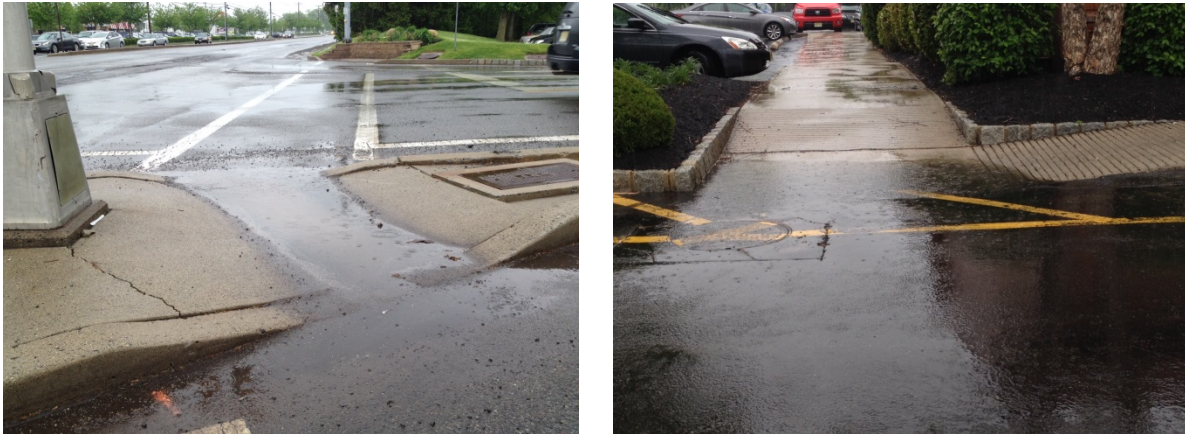
Figure F-12 (Pictures of Puddle Located on a Flush Ramp Condition)
