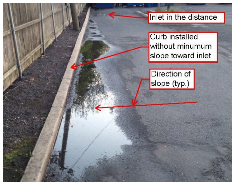
Figure F-4 (Picture of Curb Installed Without Minimum Slope)
